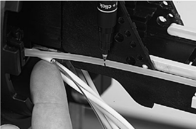
5.3.2 Mark the FOPT 20 mm measured from the end of the loose tube.
